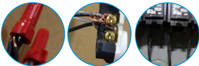
Improper solid wire connection. Improper stranded wire connection. Improperly torqued circuit breaker lugs.
